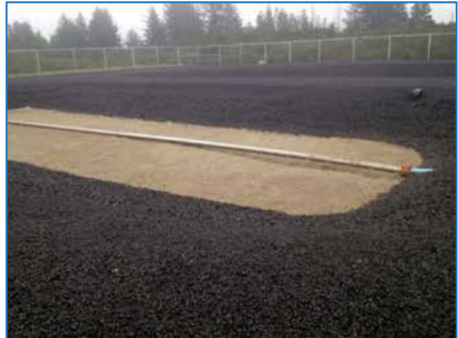
Figure 2.1 Camp Rilea Rapid Infiltration Basin
